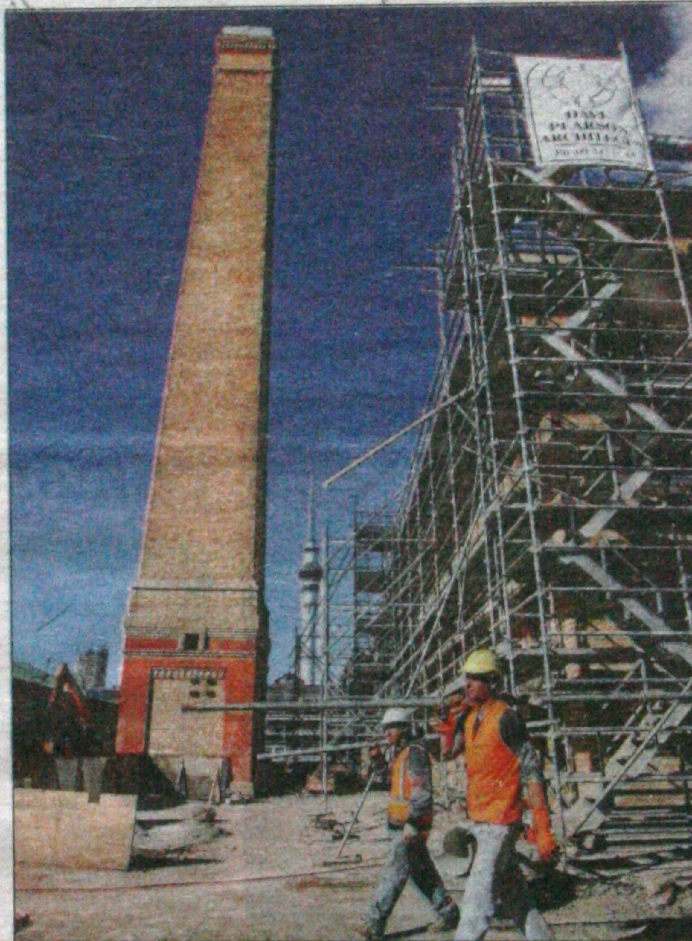
Complete revamp: Fresh life is being pumped into Auckland's Victoria Park Market which will soon be home to 80 retailers. Pictured are workmen Beto Lozada, left, and Eduardo Dos Santos.
